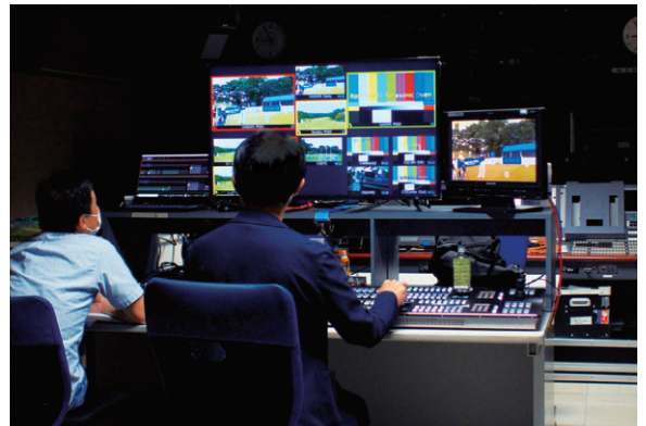
▶ Using the Kairos Control (control panel) for live streaming supported with a multi-view screen in the MBS control room
