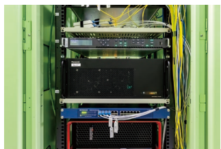
▲ Kairos Core (center rack) directly connected to the IOWN APN at the data center
