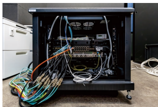
▲ SDI-to-IP converter (lower rack), integrated with network devices
